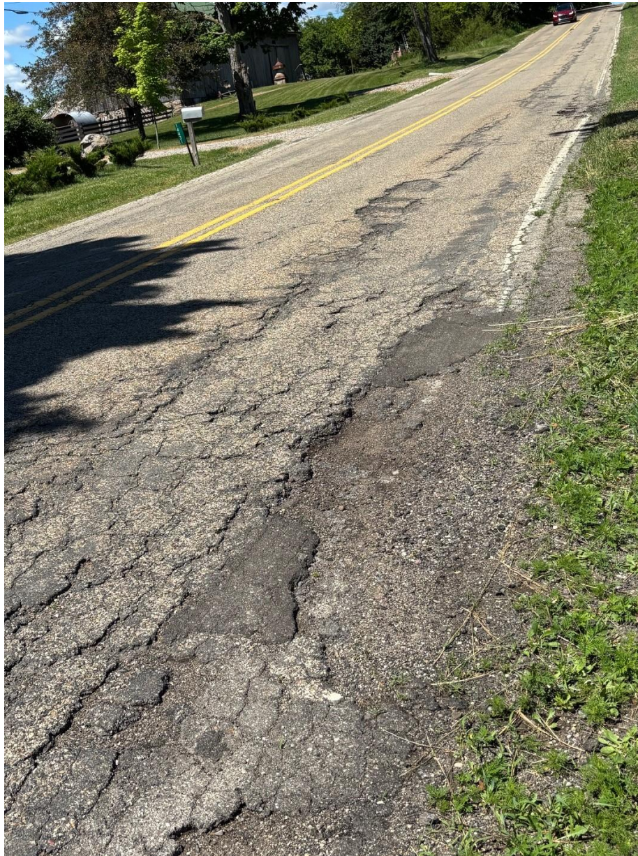
Current condition of Horning Road
